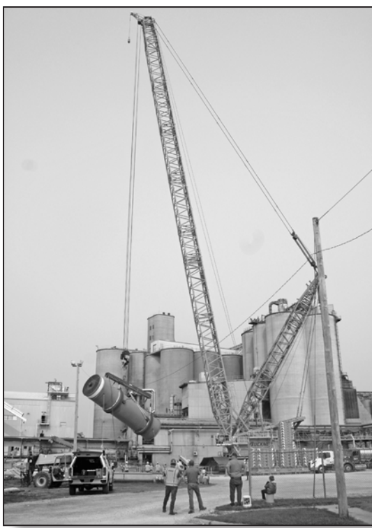
Those around town had their eyes to the sky throughout July as a giant crane dominated the skyline of Eagle Grove. It was used in conjunction with several projects, but its main purpose was to install a new rotary beam conditioner at AGP. (Photo by Edward Lynn)
