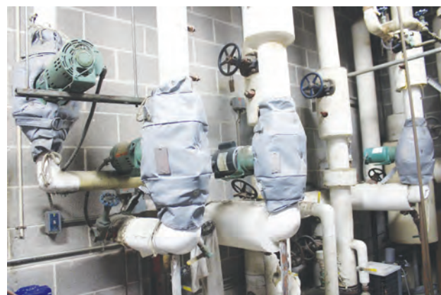
The school's water pipes
