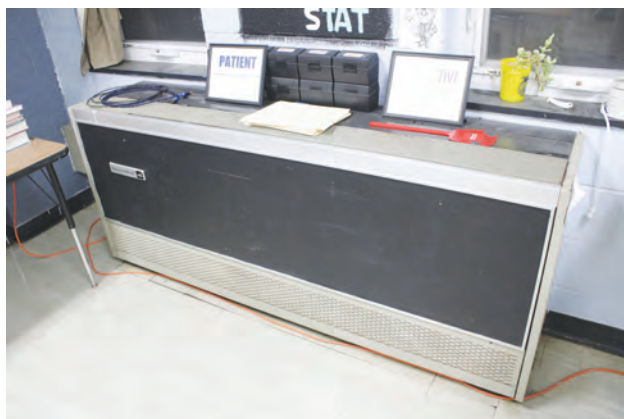
One of the nearly 60-year-old heaters.
