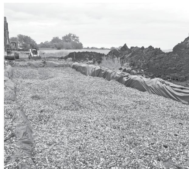
Woodchip bioreactor installation in Buena Vista County June 2019. (Photo: Iowa Learning Farms)
