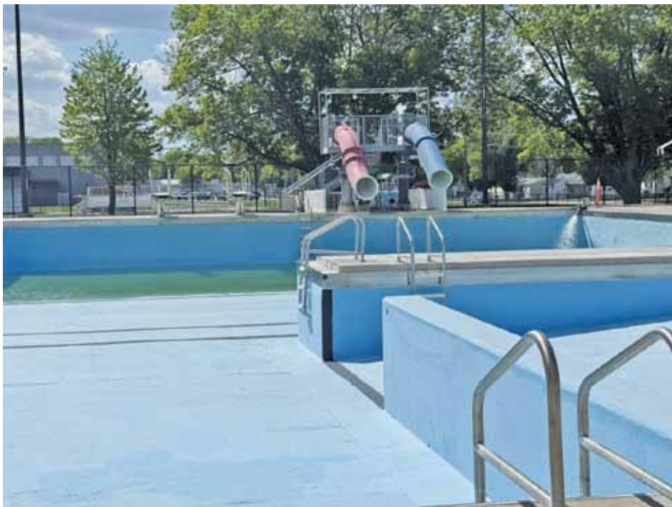
It was shared during the latest Clarion City Council meeting that the Clarion Aquatic Center is experiencing a mysterious leak. Above is a photo of the pool being filled on May 13, 2025, shortly before it was found to be leaking. (Photo: Amanda Rink)
