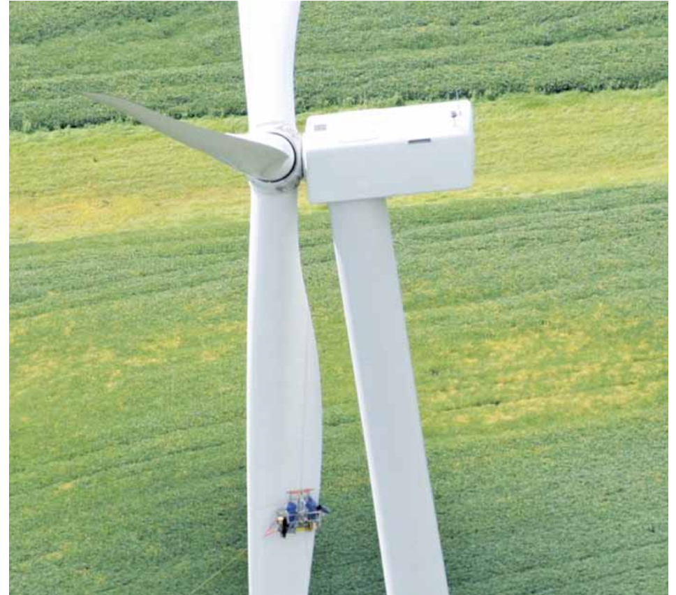
Work being done on a large windmill east of Clarion. I would think this is quite challenging.
